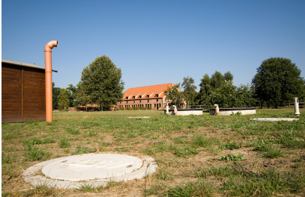
On the pasture behind the brewery (in the background) are to be found the 11 tanks belonging to the wastewater treatment plant as well as the old equipment hut, which today accommodates the complete plant control.
