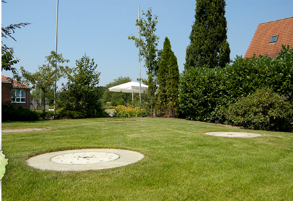
It is about 50 meters from the central drain in the cellar of the clubhouse out to the tanks of the AQUAMAX® XL-1-75 PT (Photo above). A high performance pumping station here takes on the transportation of the wastewater.
