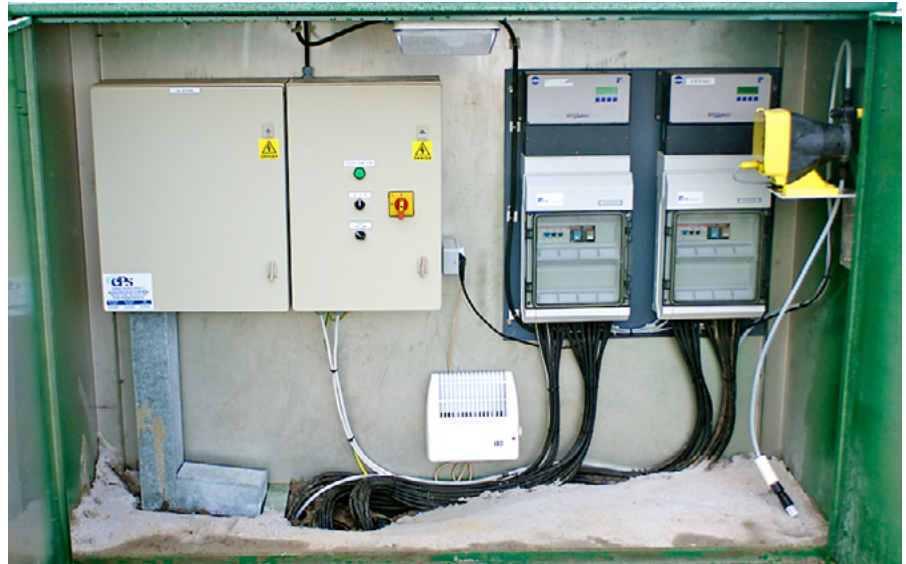
Well-arranged: the control system of the AQUAMAX® PROFESSIONAL XL-2 250.
