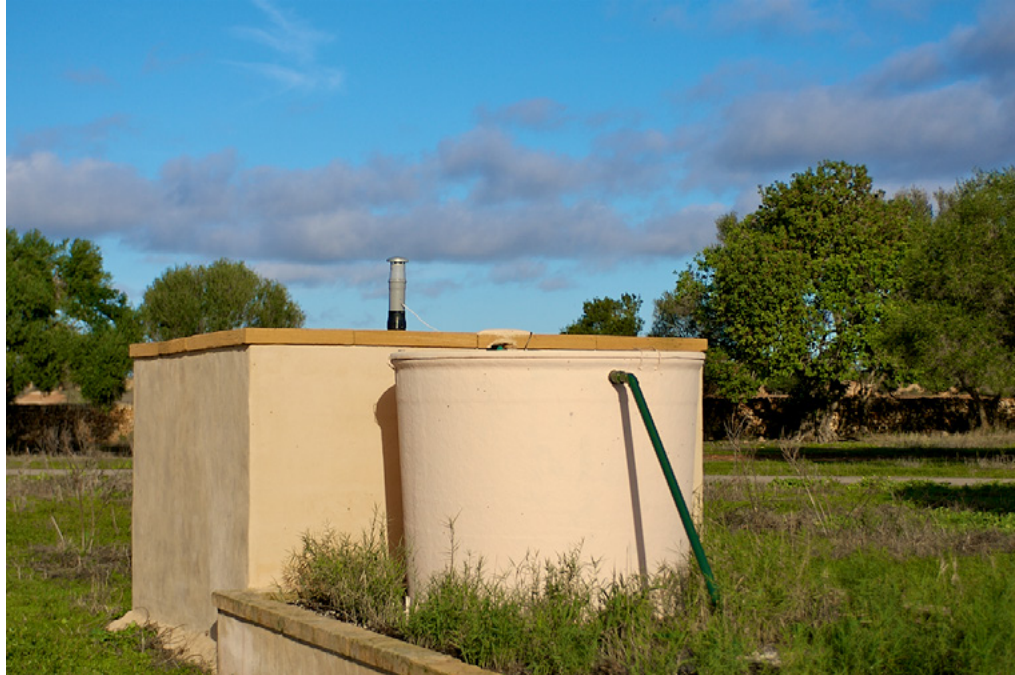
The new wastewater treatment plant at Finca S'Atalaia.
