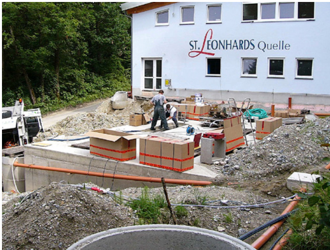
The SBR tanks, the sludge store and the buffer tank (below) were built directly next to each other in front of the new St. Leonhardsquelle production and administration building of.
